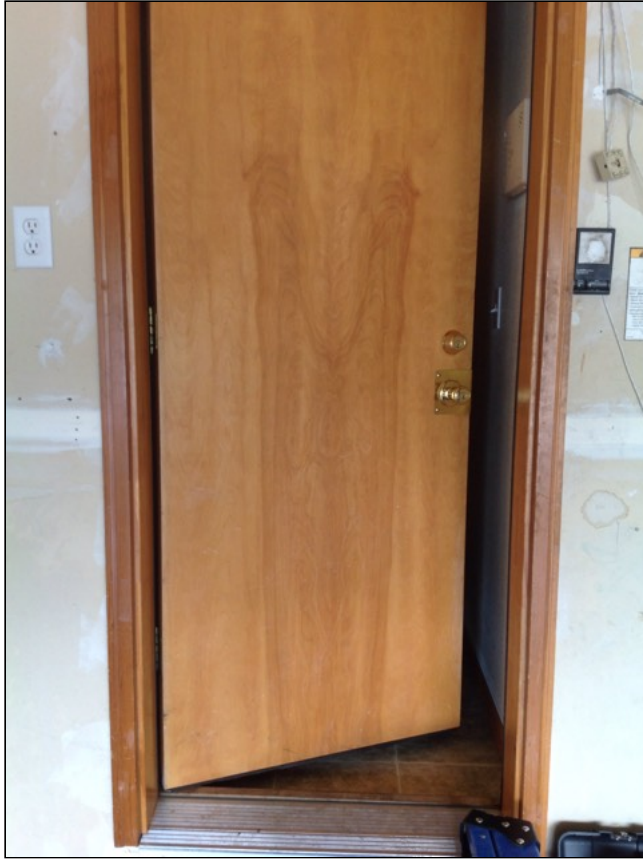
9.4 Item 1(Picture) Not self-closing. Recommend replacing to self closing hinges for safety.
