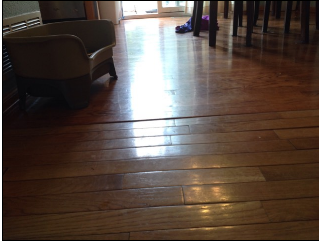
3.3 Item 1(Picture) Spacing between transitions from kitchen to 1st floor living area.
