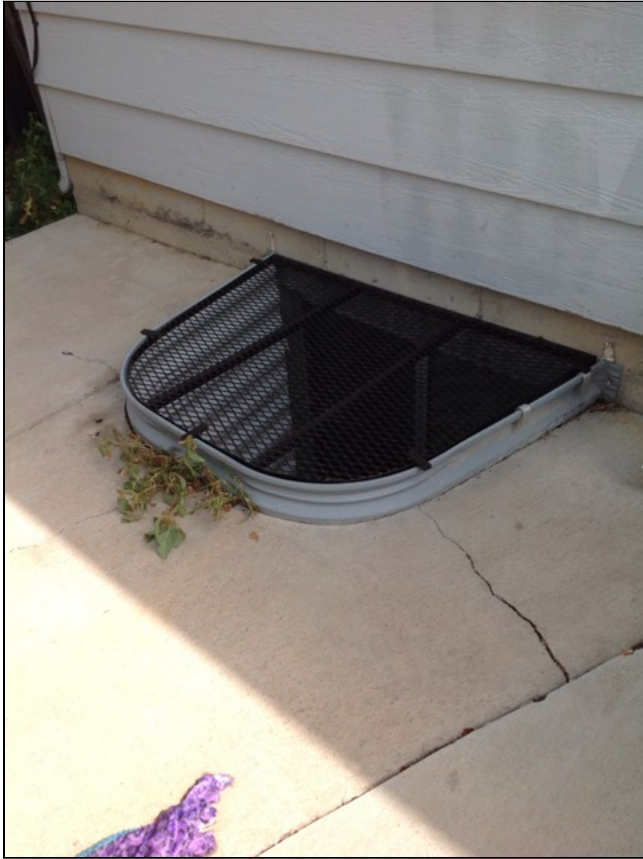
2.2 Item 1(Picture) Window well with vegetation, left side from rear of house.
