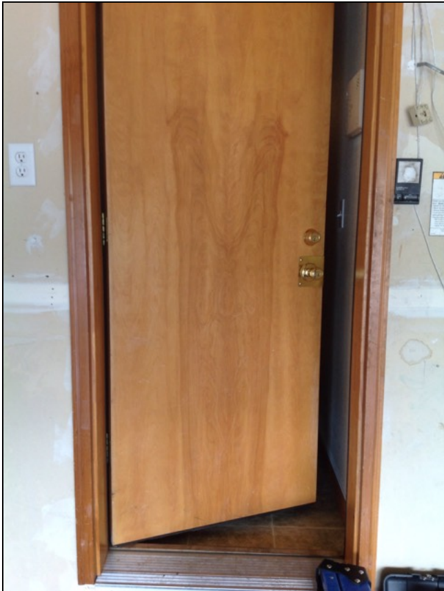
9.4 Item 1(Picture) Not self-closing. Recommend replacing to self closing hinges for safety.
