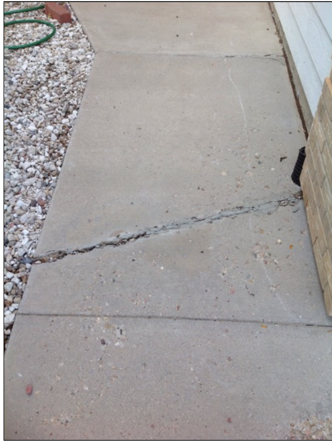
2.4 Item 6(Picture) Sidewalk to the left side of house uneven, can be a trip hazard. A fall or injury can occur if not corrected if not corrected and further erosion or deterioration can occur if not corrected a qualified contractor should expect every day or as needed
