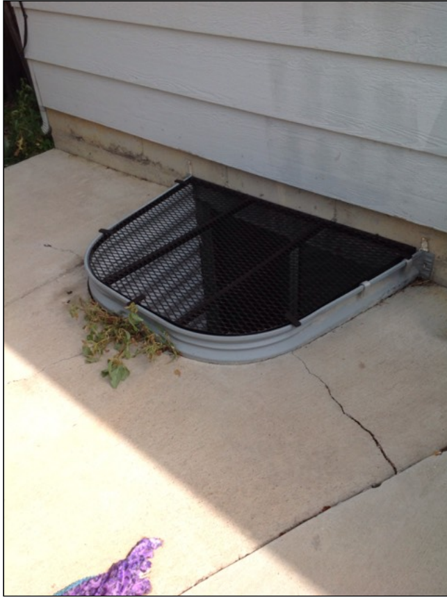
2.2 Item 1(Picture) Window well with vegetation, left side from rear of house.
