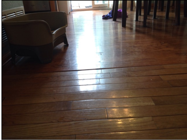
Spacing between transitions from kitchen to 1st floor living area.
