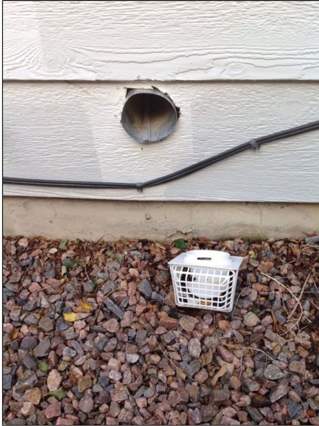
2.0 Item 3(Picture) Ventilation exhaust not in use. Recommend remove and sealing exterior wall
