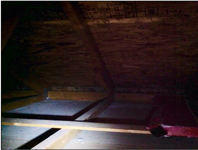
1.2 Item 3(Picture) Space above garage. No flooring insulation.
