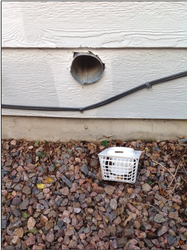
2.0 Item 3(Picture) Ventilation exhaust not in use. Recommend remove and sealing exterior wall
