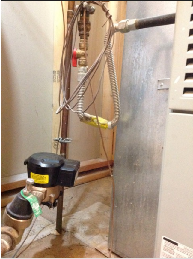
5.5 Item 1(Picture) Main fuel source shut off valve. Red valve. Utility room in basement level.
