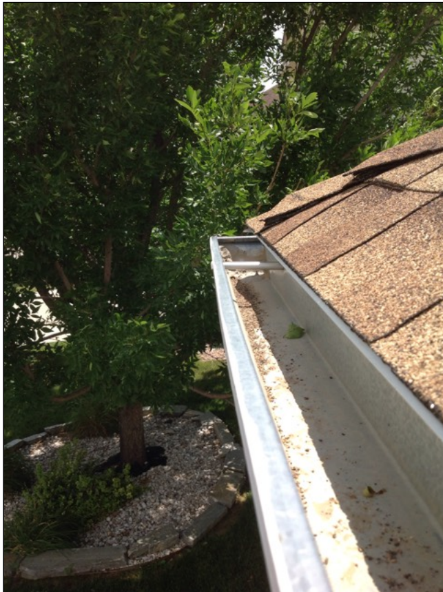
1.1 Item 1(Picture) Drop edge flashing present on all gutters.
