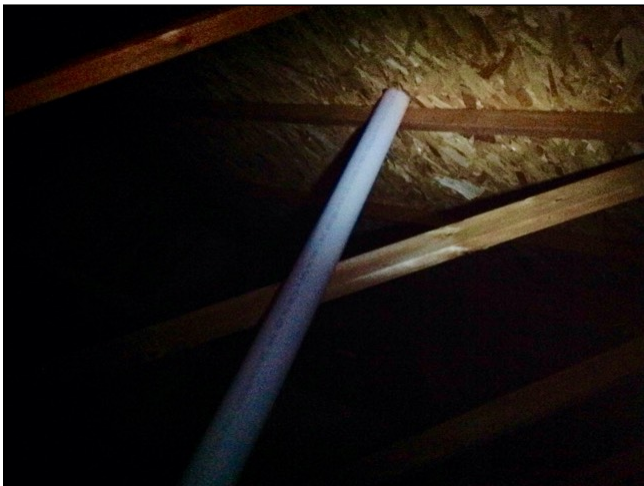
1.2 Item 5(Picture) Plumbing vent pipe.
