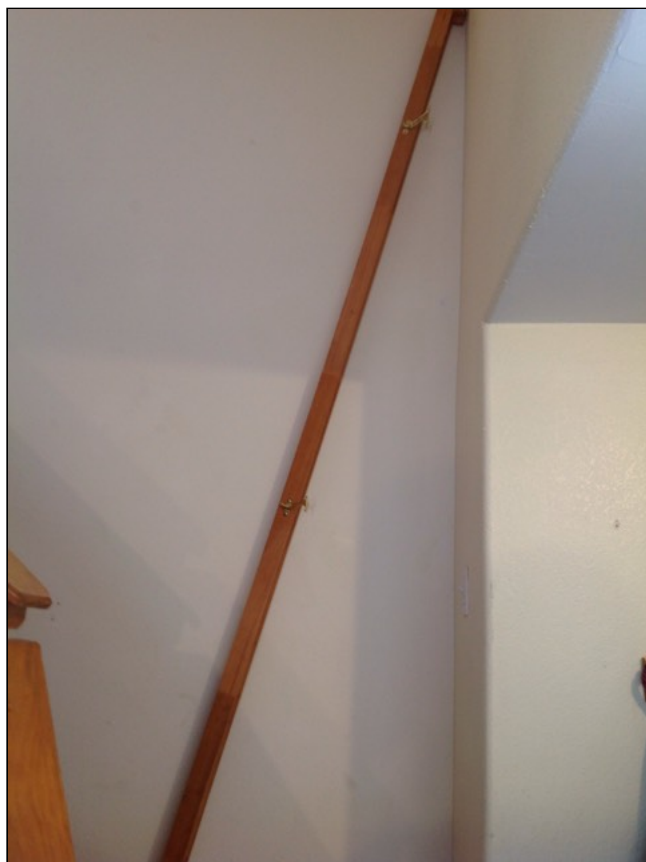
8.3 Item 1(Picture) The hand/guard rail for the second story stairs missing. A fall or injury could occur if not corrected. A handrail should be installed for safety.
