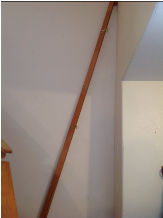
8.3 Item 1(Picture) The hand/guard rail for the second story stairs missing. A fall or injury could occur if not corrected. A handrail should be installed for safety.
