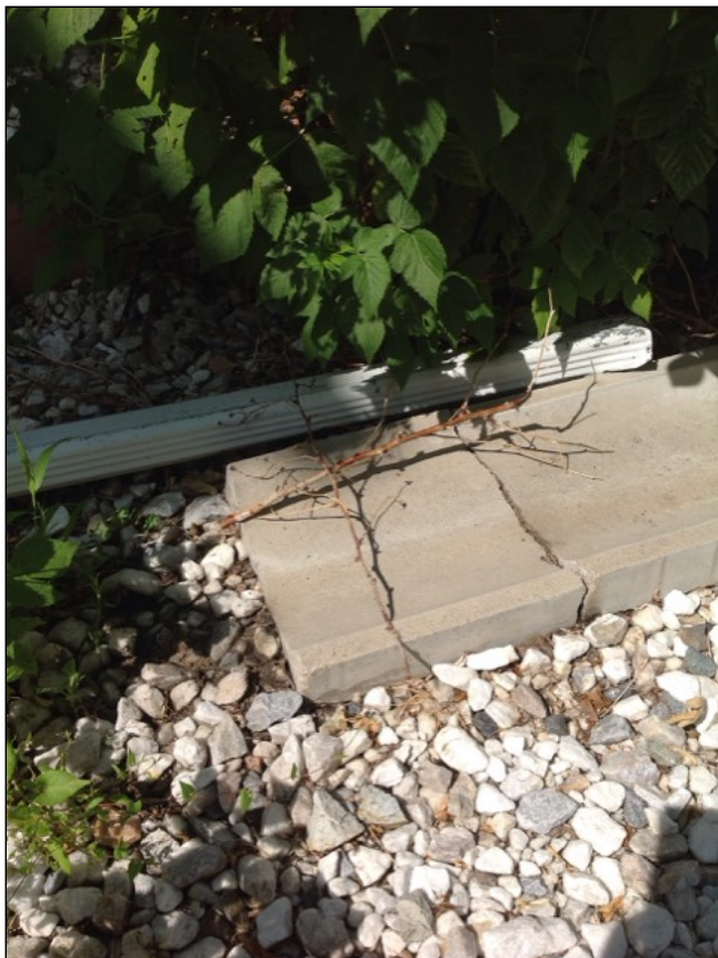
The gutter splash-block at the front left corner of home has cracking. Replace, reinstallation or use of gutter extension replacement as desired.
