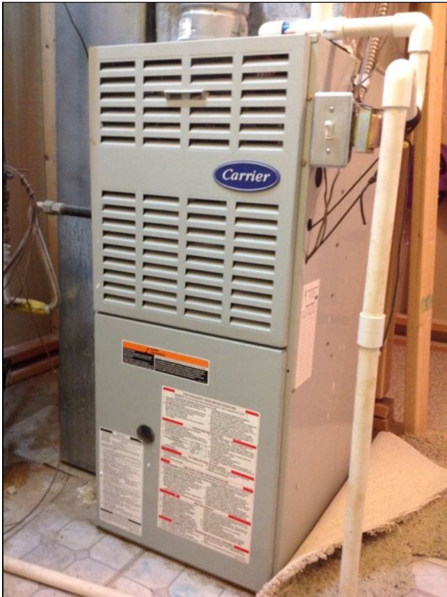
4.0 Item 1(Picture) Located in utility closet basement level
