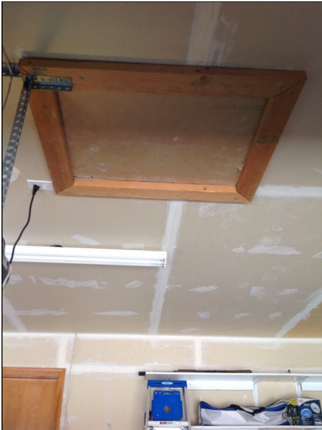
1.2 Item 1(Picture) Attic space access above garage. No flooring insulation present.
