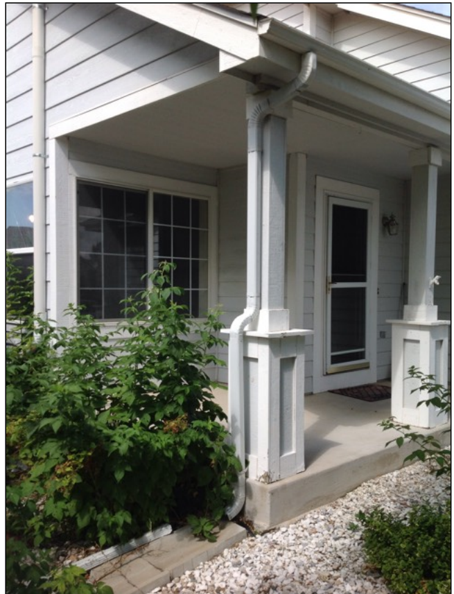
Vegetation needs to be trimmed and/or removed.
