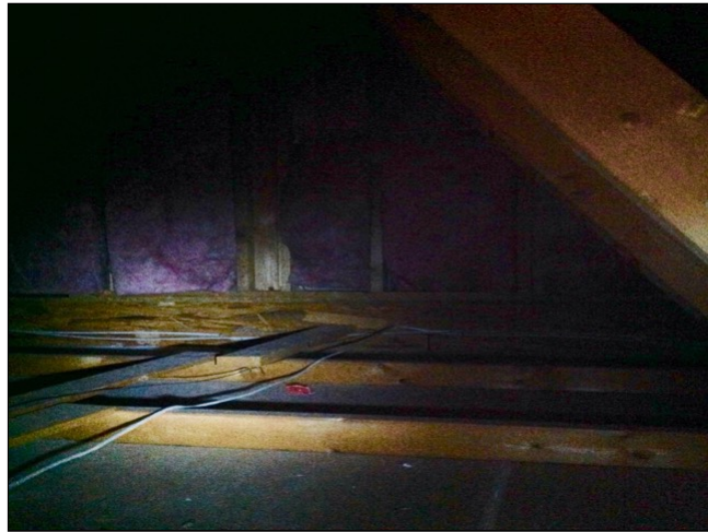
1.2 Item 2(Picture) Space above garage. No floor insulation.
