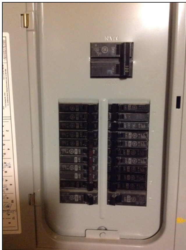
Panel located in garage; left wall. No ACFI present in panel.
