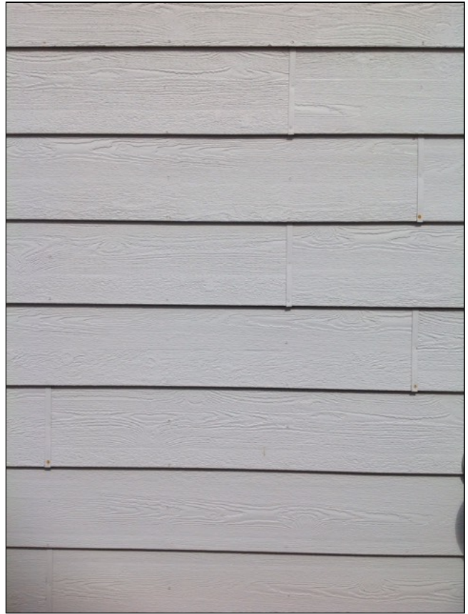
2.0 Item 2(Picture) Rusty nail heads present at left side (facing front). Repair as needed.
