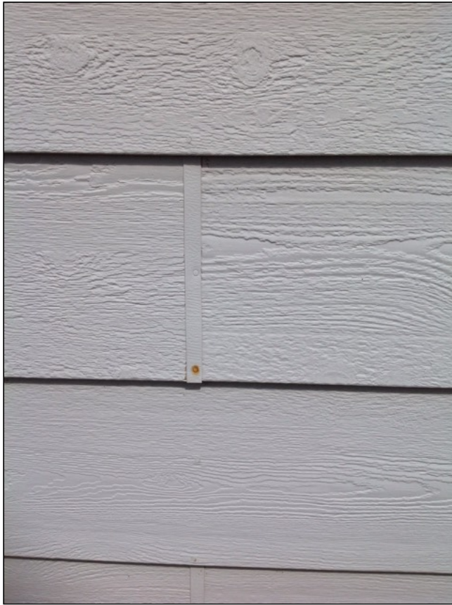
2.0 Item 1(Picture) Rusty nail heads present at left side (facing front). Repair as needed.
