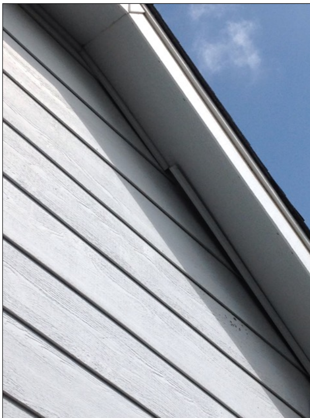
2.5 Item 2(Picture) Molding under eave at left side of house loose. Repair as needed.
